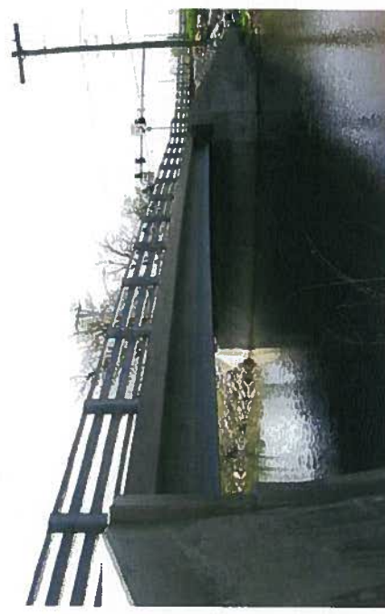
Reference: Bridge. Federal Highway Administration, Route 31, Lyons, New York. Construction of Field-Cast Ultra-High Performance Concrete Connections. Web. 9 Mar. 2016.
