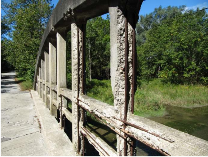
Plate 18: Detail of damaged handrail and vertical members.
