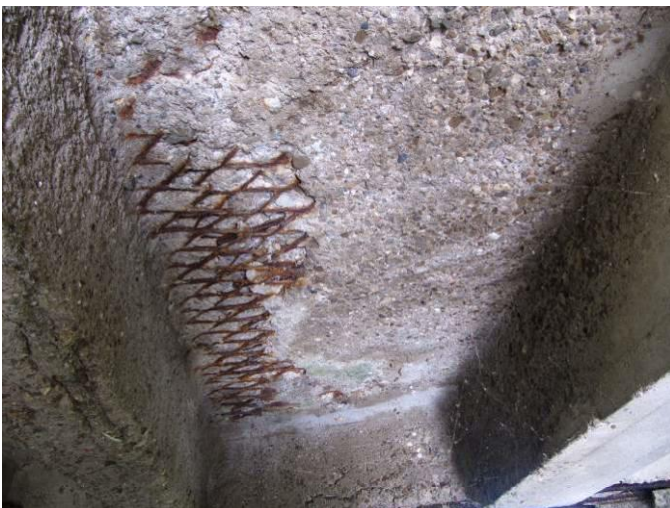
Plate 8: Detail of spalling soffit
