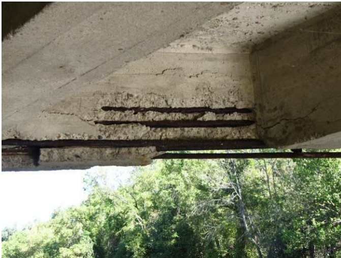
Plate 9: Detail of exposed rebar.
