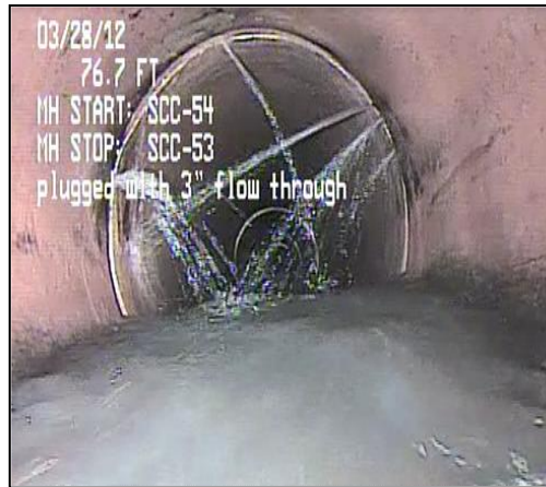
CCTV Inspection showing Infiltration/Leakage in a pipe
