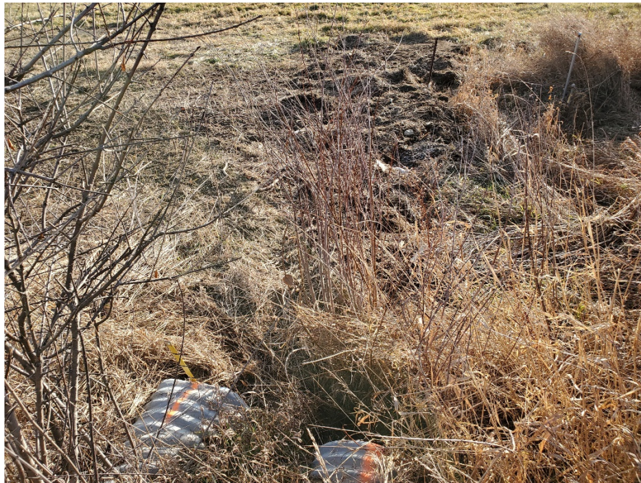
Photograph taken facing downstream (south) of Kirby Road. Double CSPs were noted crossing Kirby Road.
