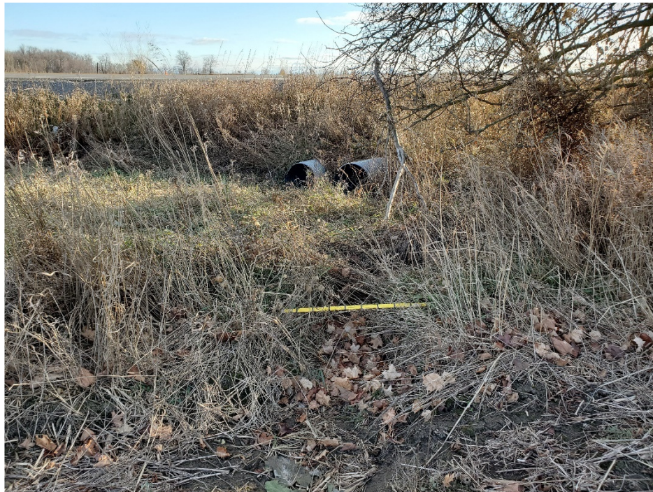
Photograph taken facing downstream (south) towards the double CSPs at Kirby Road. There was a small defined channel between the agricultural field and the CSPs.
