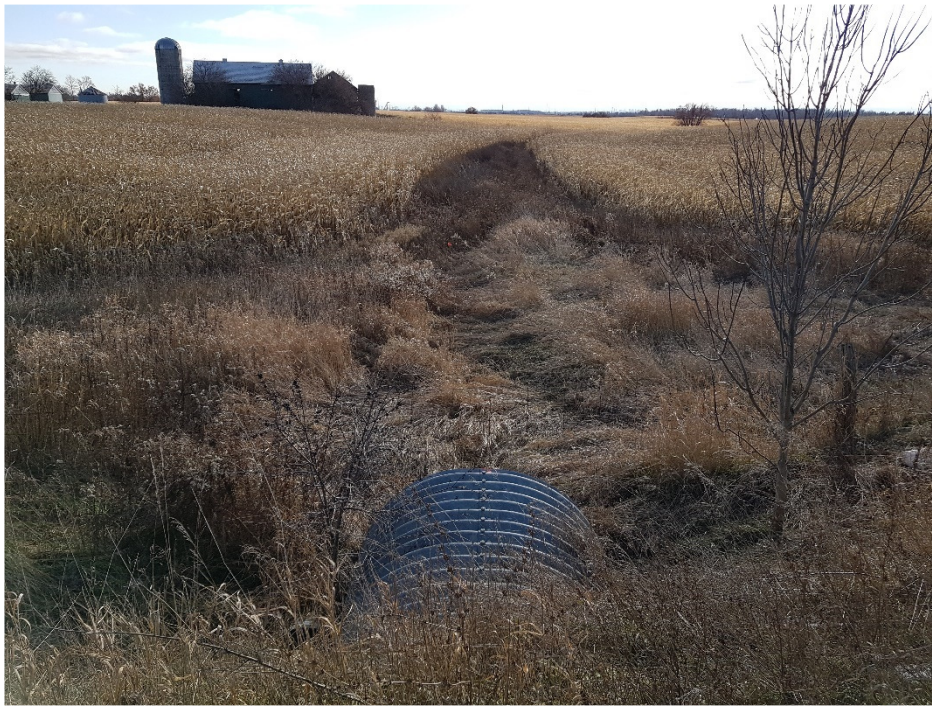
Photograph taken facing downstream (south) of Kirby Road. The swale feature flowed through an active agricultural field.
