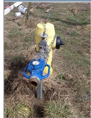
HYDRANT PREPARED FOR SAMPLING
